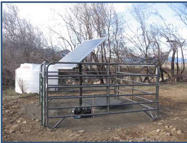
A solar stockwater system installed in the Hornbrook area as part of our Bogus Creek Grant from the California NCWQCB.
